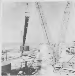
Sitting on the Ringer which allows 360 degrees rotation, the Manitowoc Crane slowly lifts tower for Hydrogen Plant.
